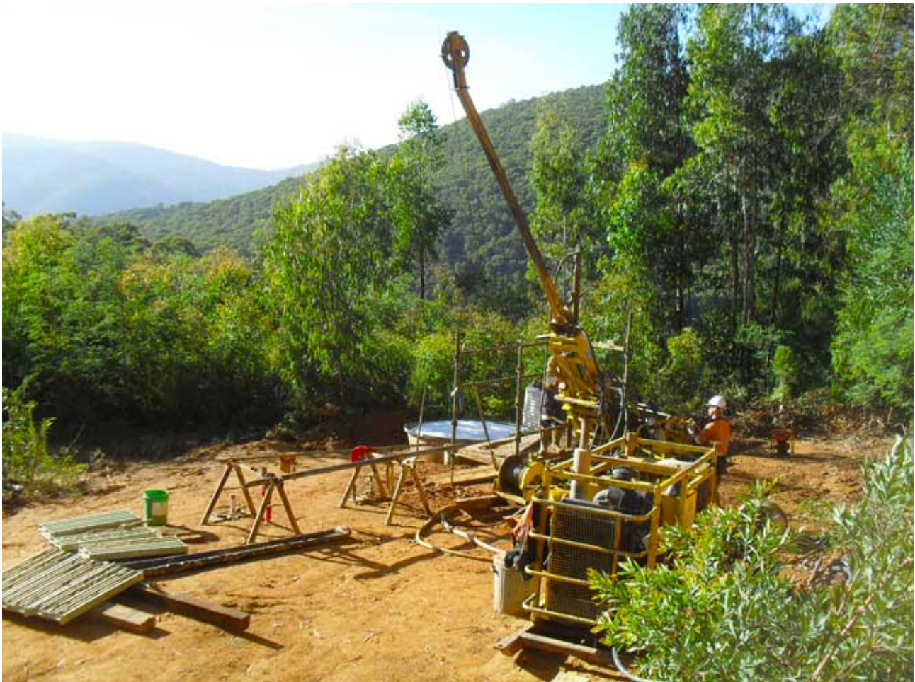
Drilling from surface of Morning Star dyke into AAA reef zone of Morning Star goldmine
