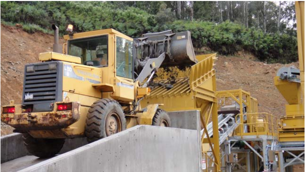
Morning Star's New Gravity Processing Plant (GPP) receives its first load of commissioning ore
